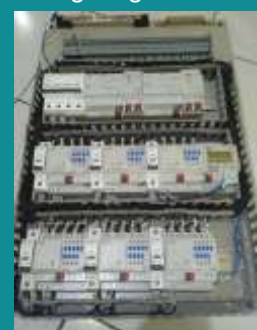
KNX Lighting automation
