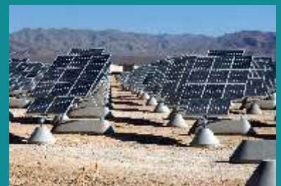
Solar Power Plant (PLTS)
